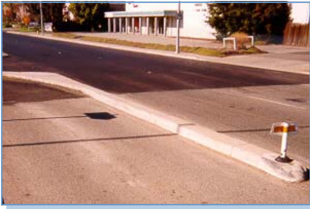
Painted concrete leads to maintenance problems
