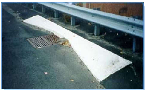
A water control inlet "bow tie"
